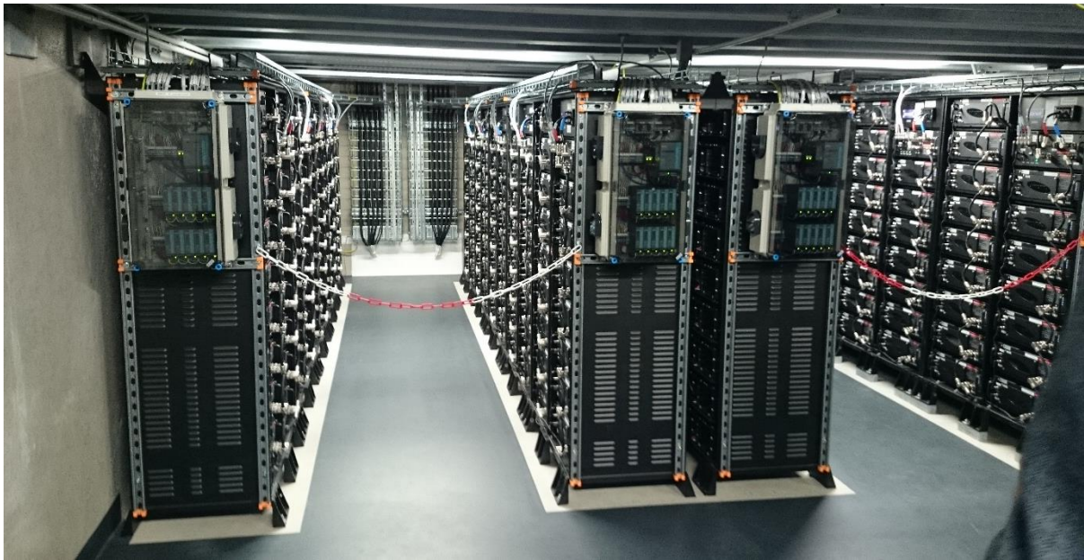
Figure 3.5: Interior view a battery storage power plant [64].
