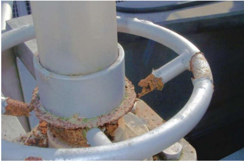
Figure 6. The valve handle on the clarifier displays significant corrosion. (Stephenson & Kumar, 2009).
