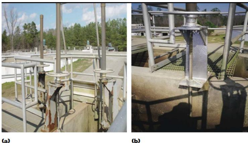
Figure 7. The a) initial and b) final states of the valve-operator stands at a wastewater treatment plant. (Stephenson & Kumar, 2009).
