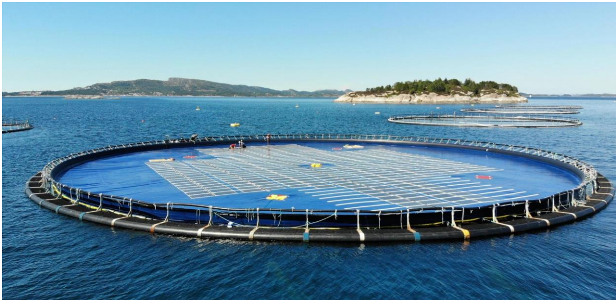
Figure 4.2: A floating solar system from Ocean sun SA [26] .
