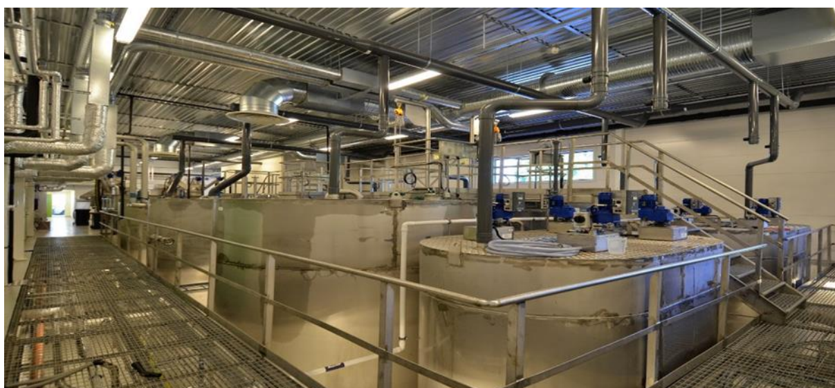
Figure 1 Bø sewage wastewater treatment plant (Skarweld AS, 2014).
