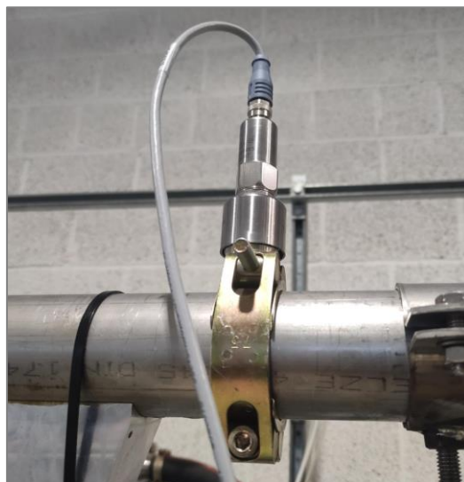
Figure 3.4: Clamp-on HS-100 accelerometer sensor fitted on horizontal pipe in USN rig
