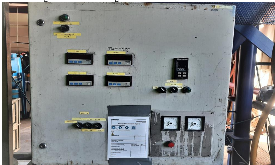
Figure 3.9: Pneumatic control panel.
