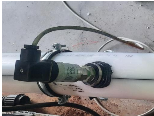
Figure 3.8: Pressure transducer along the pipeline
