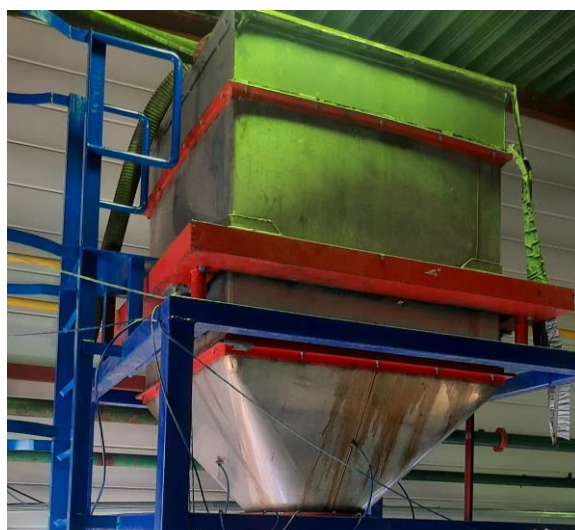
Figure 3.4: View of the receiving tank.
