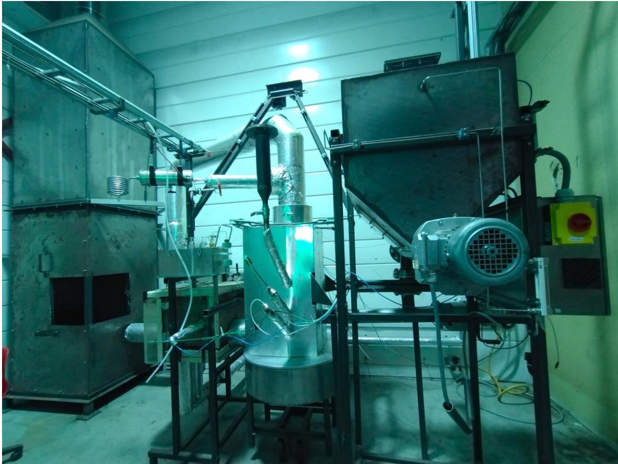
Figure 4-4. BFB gasification reactor at USN, Porsgrunn
