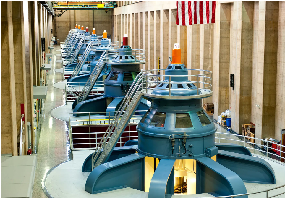
Figure 3.5: Generator unit at typical hydropower plant [41]
