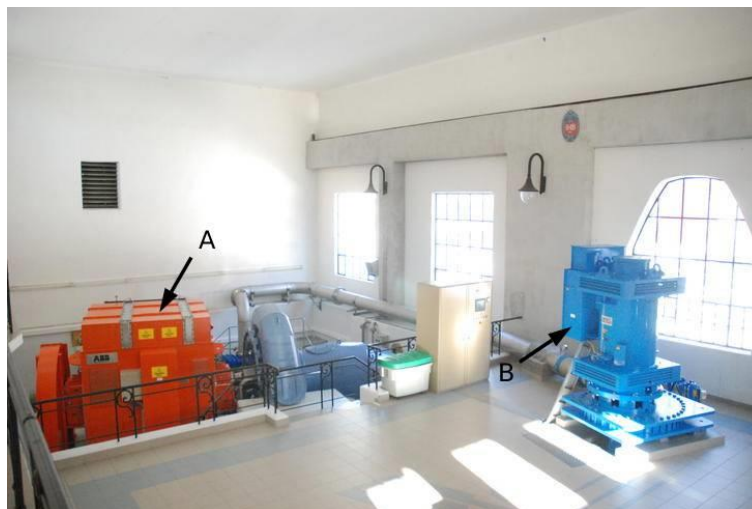
Figure 1.1: Generators in the Hogstad hydropower plant. A: 9 MW generator, B: 0.6 MW generator. [10]
