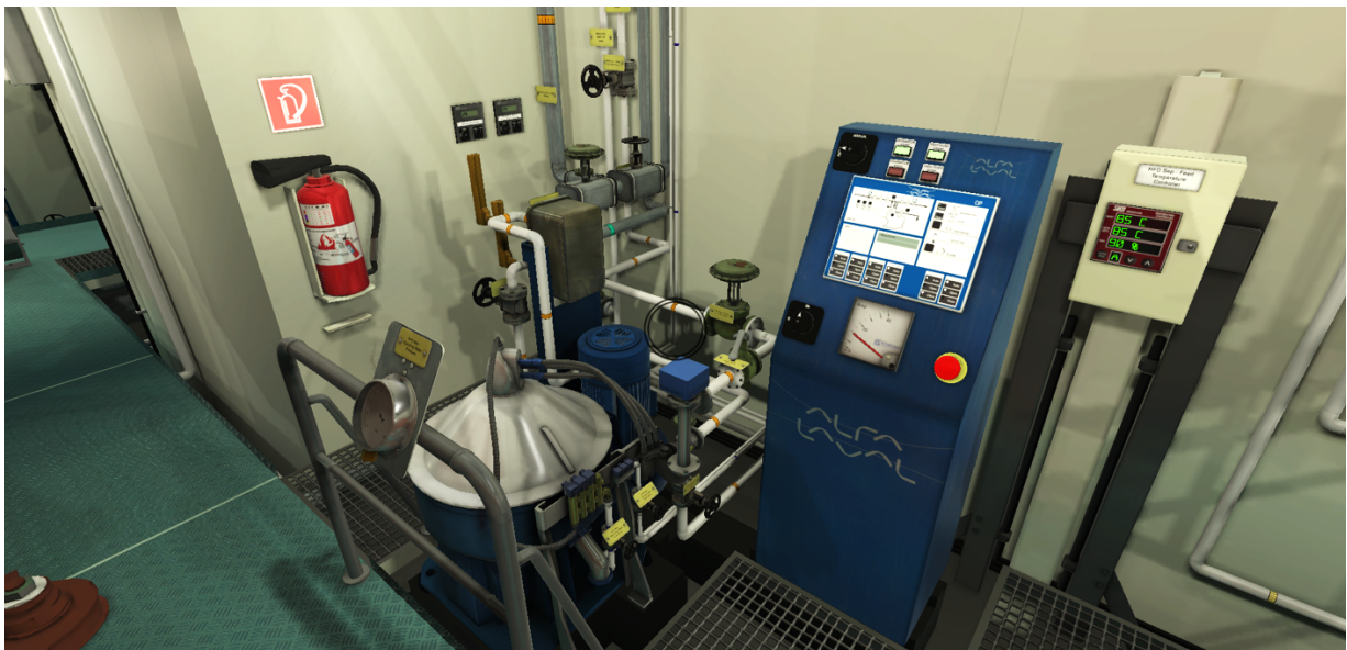
Figure 14: Fuel oil separator as viewed through the monitor of the 3D virtual reality desktop simulator
