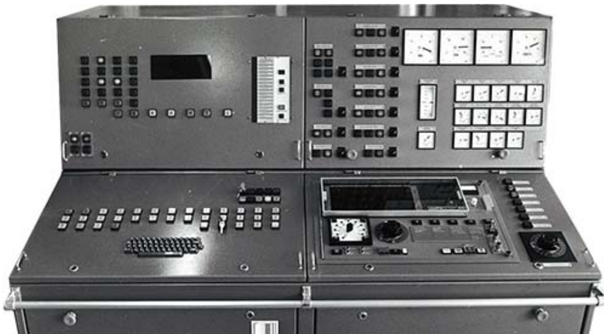
Figure 3: The Norcontrol diesel engine simulator delivered to Trondheim Maritime College in 1978 (Kongsberg Maritime, 2019b)
