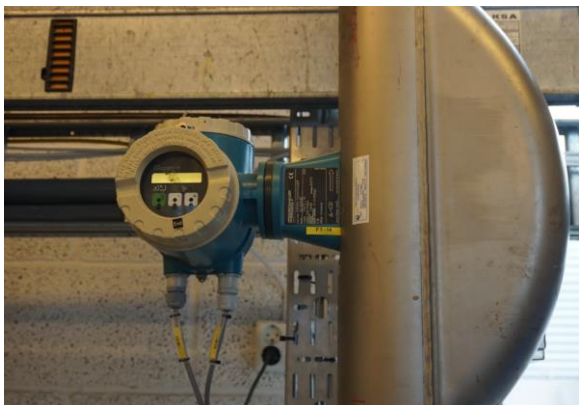
Coriolis flow meter (Promass 63)
