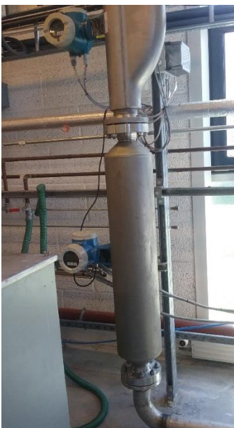
Figure 2B- 3. Position of Old and New Coriolis flow meter
