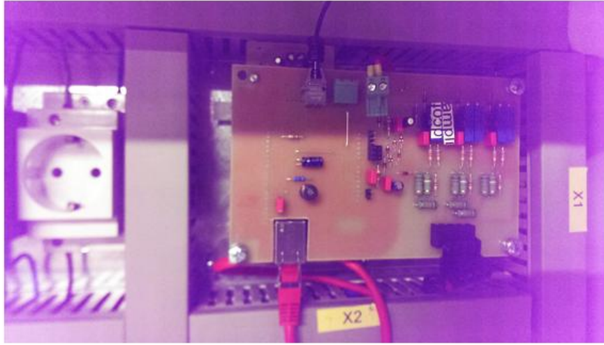
Figure 8-3: Measurement Electronic Board Mounted in the Power Cabinet with Arduino Board Connected At the Back.
