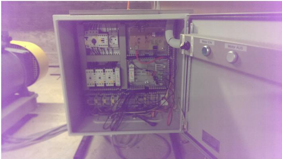
Figure 2-2: Small Scale Power Grid Connected to the Output of the 60Hz Machine.
