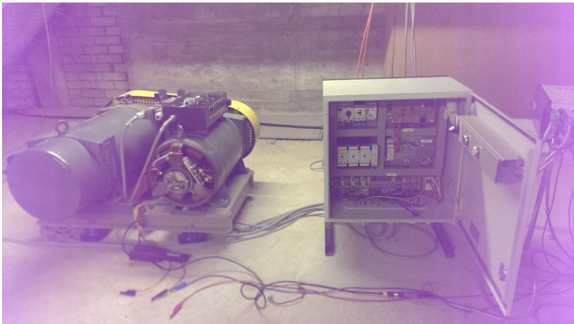
Figure 2-3: Mechanically Coupled 50/60Hz Machine (Frequency Transformer Units) Connected to the Power Grid.
