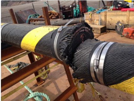
Figure 15 Power cables at FORCE. Source: FORCE
