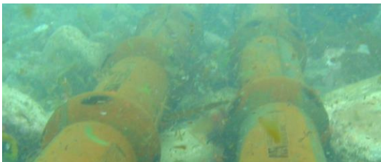
Figure 16 Power cables with iron protection EMEC. Source: EMEC
