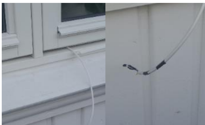
Figure 2-20 Outside sensor placement, sensor 7 seen in image
