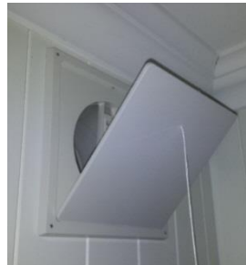
Figure 2-23 Ventilation locations, living room vent seen in image
