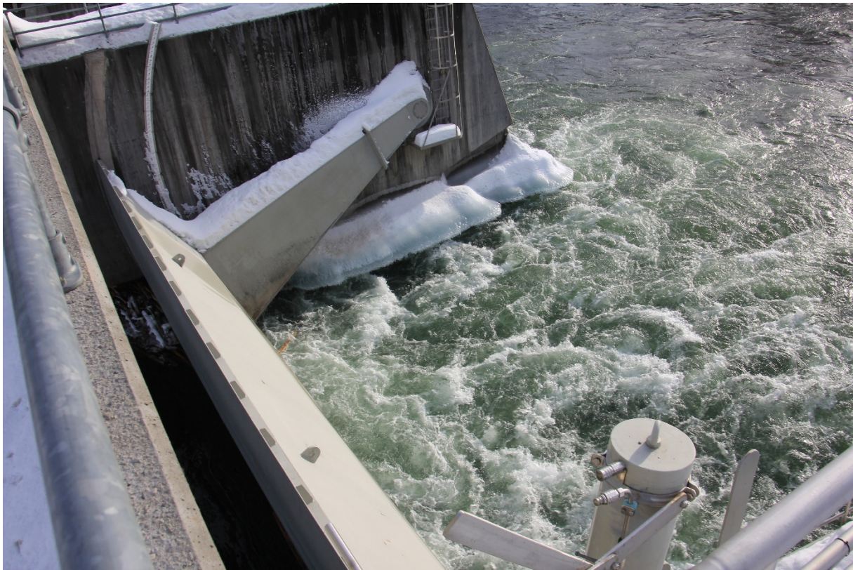
Figure 2-5: The segment gate of Grønvollfoss Power Plant.
