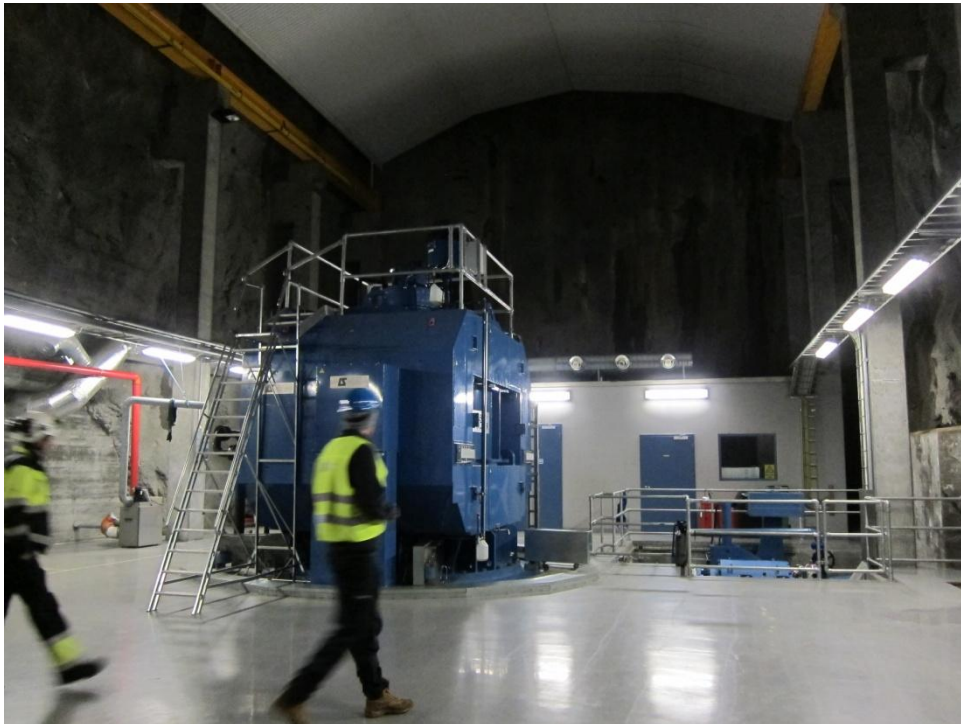
Figure 3-3: Grunnåi Power Station with its generator
