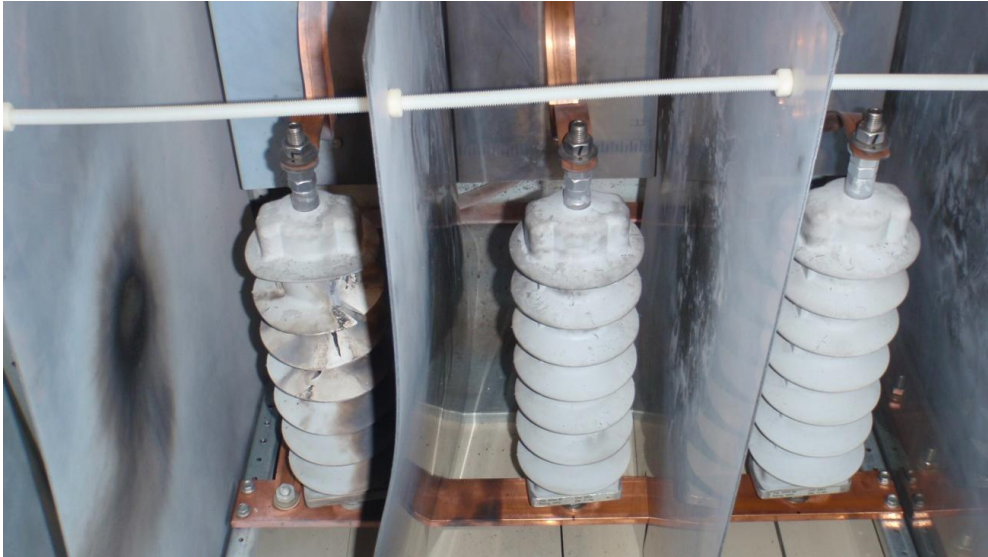
Figure 3-9: Broken surge arrester
