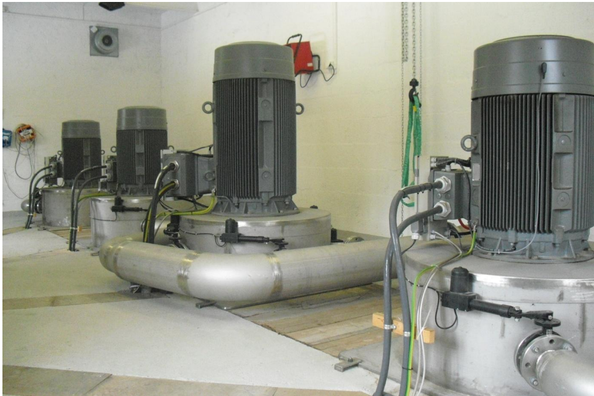
Figure 3-6: The four generator units in Sagbekken 2 and 3
