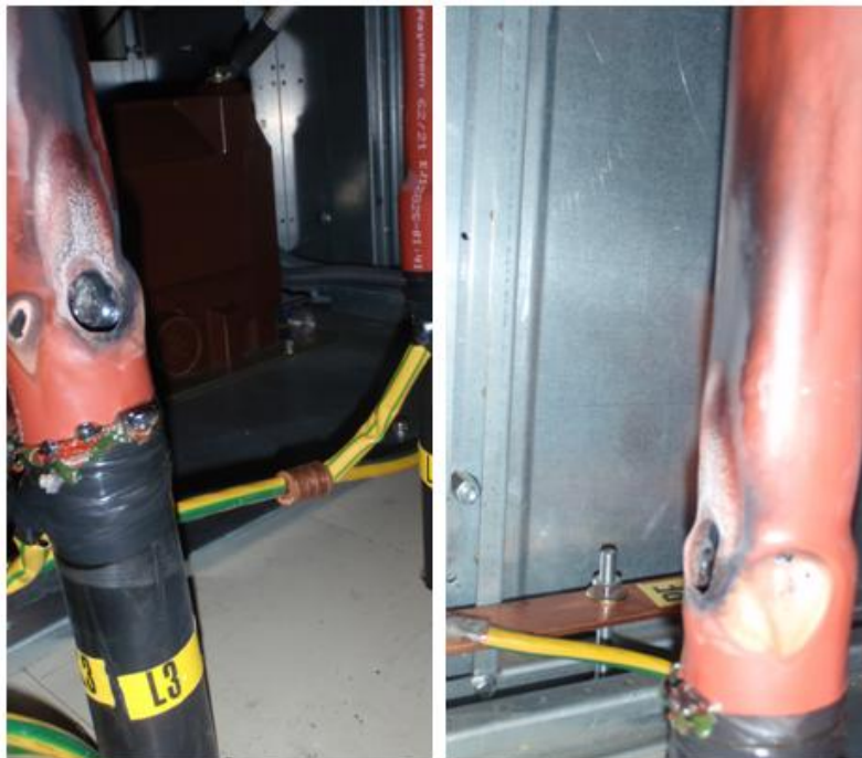
Figure 3-8: Phase to ground fault on end termination of TSLE cable
