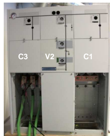
Figure 1: Front view of the test object with two cable modules (C1 and C3) with LBS and a transformer T-off (V2) with a vacuum circuit breaker.
