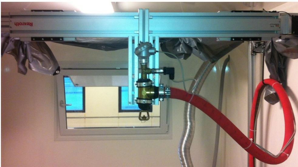
Figure 3.5: Positioning system with fire water nozzle applied.
