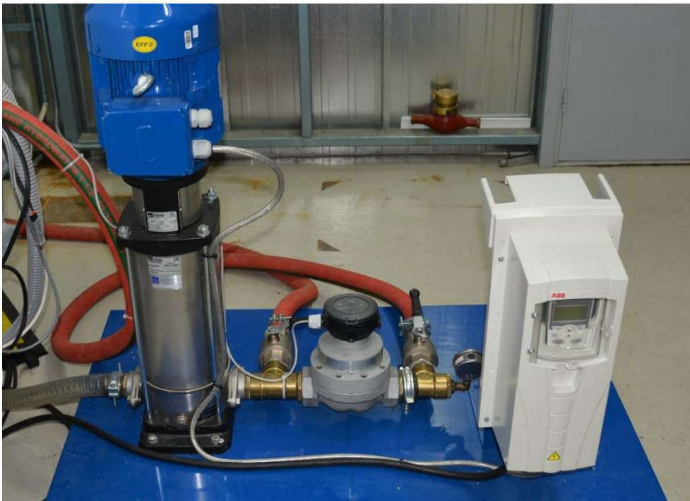
Figure 3.7: Pump and frequency converter on moveable skid.
