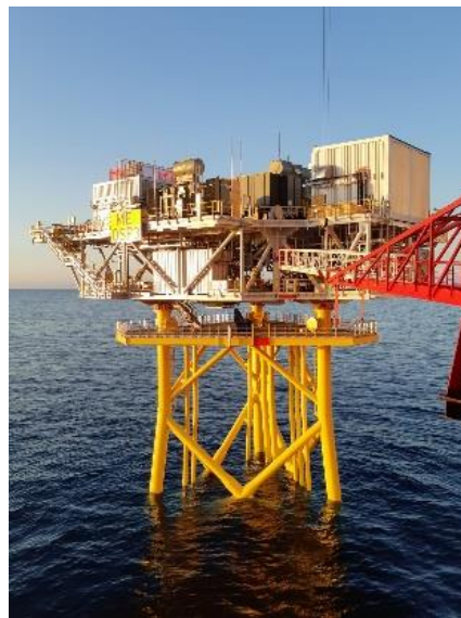
Figure 3 Offshore Sub-Station Moray East (Moray East OWF, 2020)
