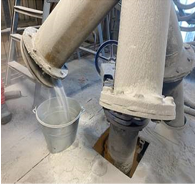
Figure 3.2 Basement dust collecting from the floor
