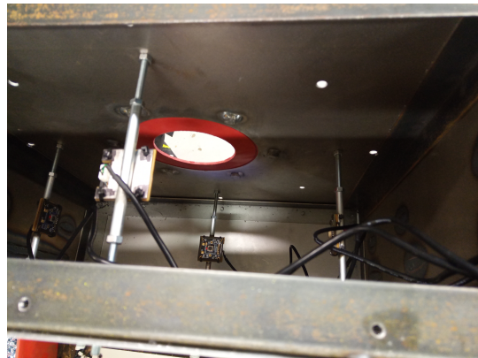
(b) The cameras are installed into the metal frame.
