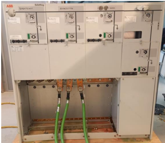
Figure 3.3: Frontside of switchgear.
