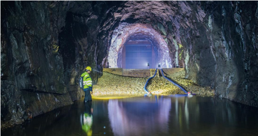
Figure 3.1: Cleaning process of a sand trap in Rosekrepp hydropower [21].
