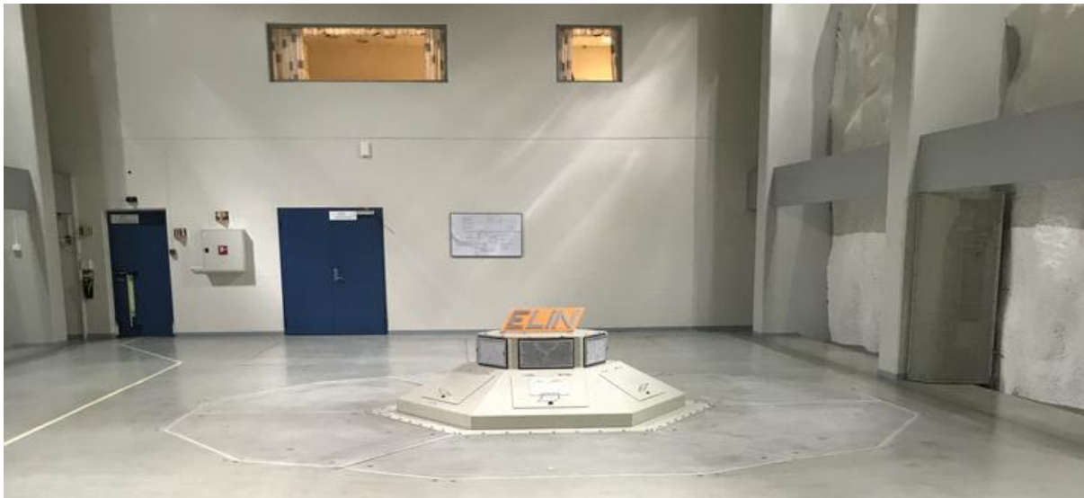
Figure 4.2: Inside of Åbjøra power station, showing the generator. [Photo: Skagerak Kraft]
