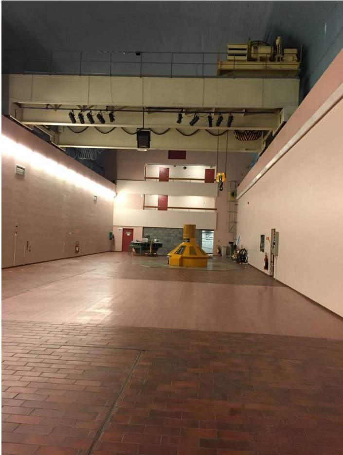
Figure 4.4: Inside of Sundsbarm power station, showing the generator. [Photo: Skagerak Kraft]
