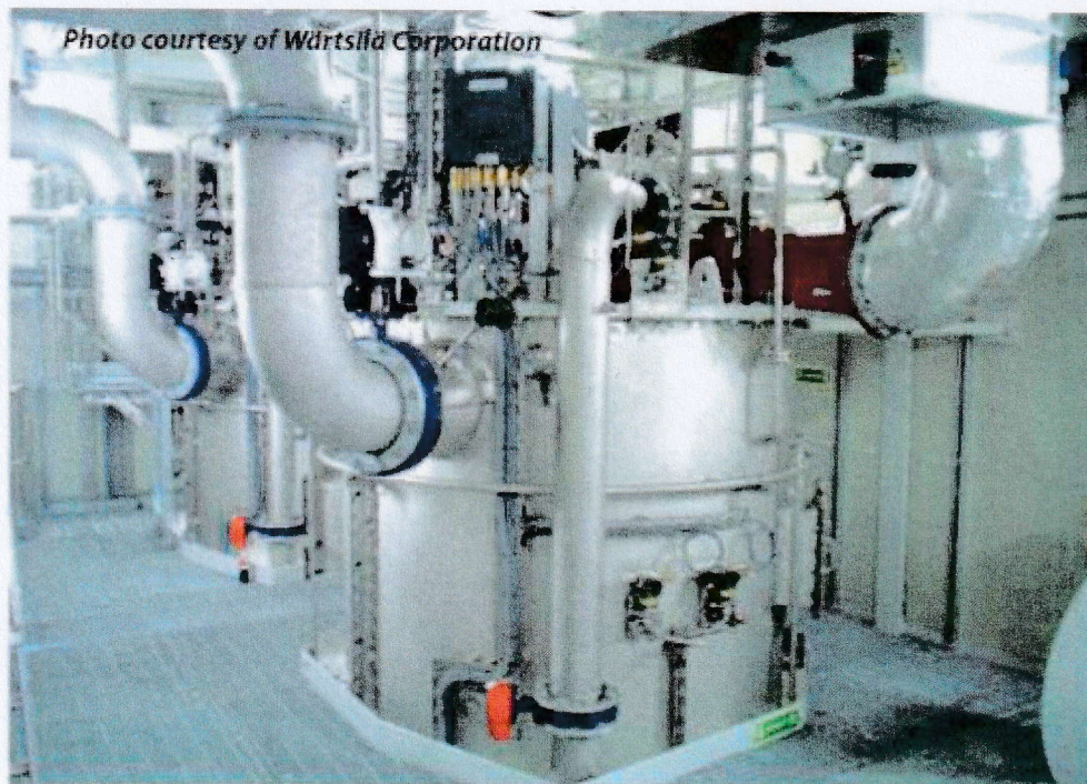
Figure 1: Inert gas generator/Boil-off gas handling equipment
