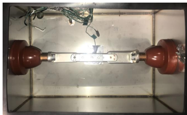
Figure 4.7 – Picture of one of the switches mounted between the bushings inside the small enclosure
