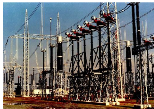
HV outdoor switchgear [5]
