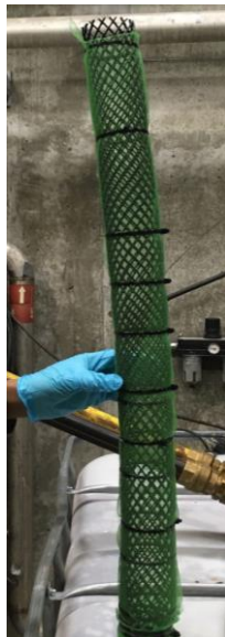
Figure 4-3: Installed solid filter mesh inside the feeding tank. The filter mesh was approximately 1.5 m long and the feed pipes were inside the mesh
