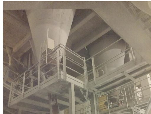
Figure 2-10: Bottom part of the two cyclones
