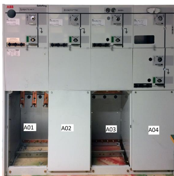
Figure 3-1: Picture of the front of the 4-module switchgear.
