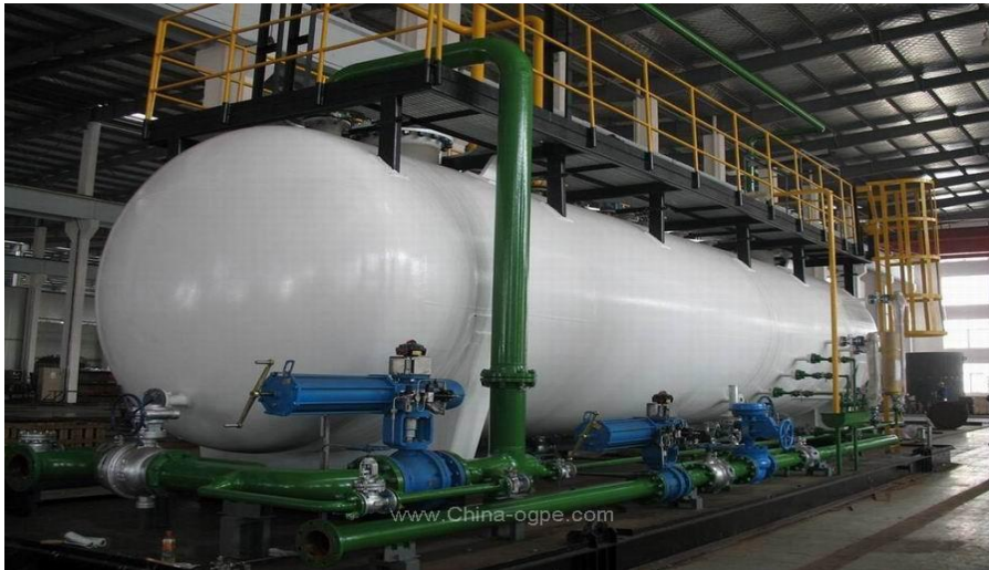
Figure 1-1 Offshore 1 st Stage separator
