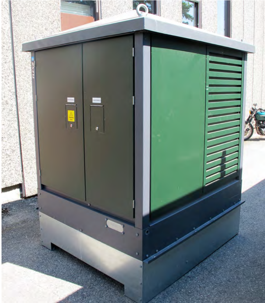
Figure 1.1: A typical substation located around Norway - This is a smaller one compared to where the switchgear that is being experimented on, it serves an illustrative purpose
