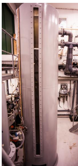
Figure 4-2: Filter in the pilot plant.
