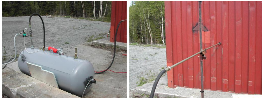
Figure 3.4 Gas storage tank and fuel supply system.
