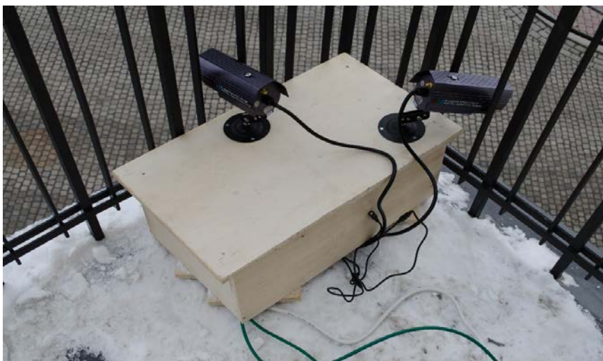
Figure 4-2 Installed cameras on the balcony and focused on two major directions
