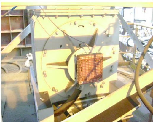
Figure 3.24: Rotary valve with air sluice
