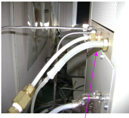
Figure 5.18: Exhaust outlet of TGA
