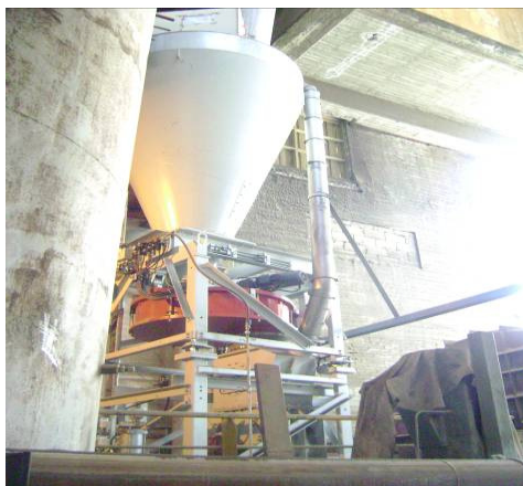
Figure 3.10: Pfister feeder system
