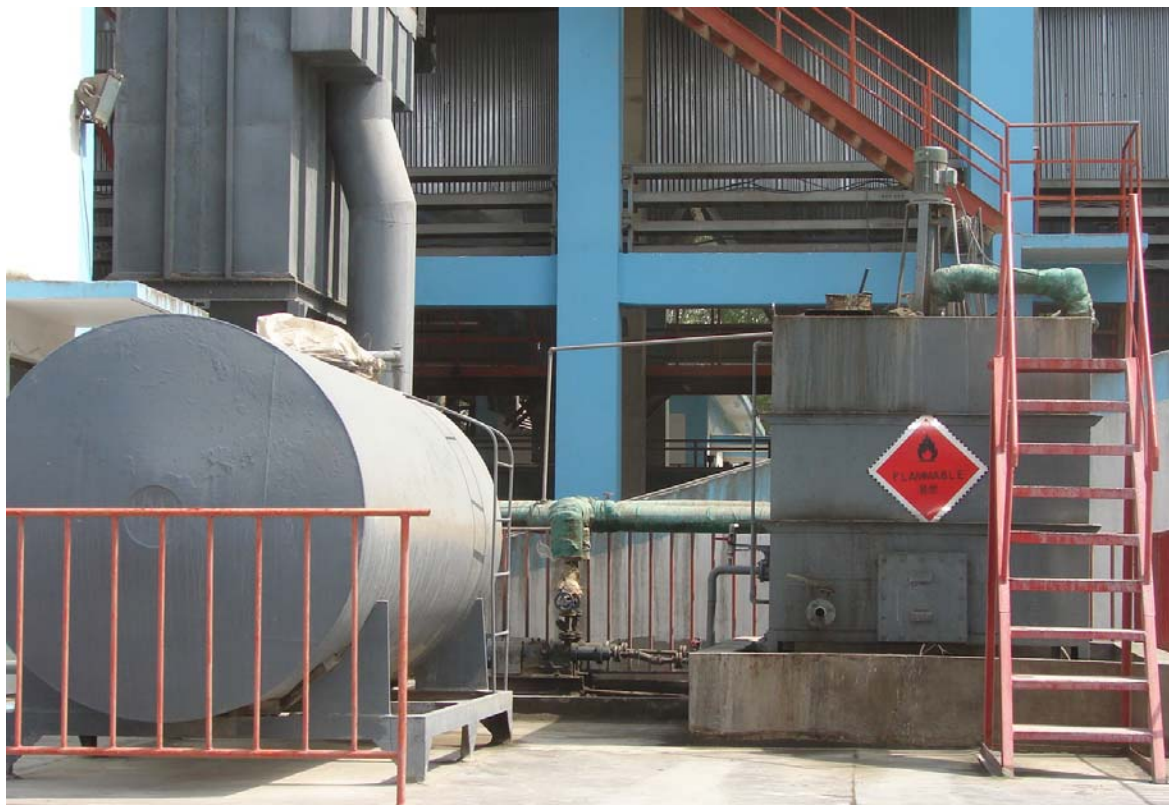
Figure 25: The real liquid disposal system.
