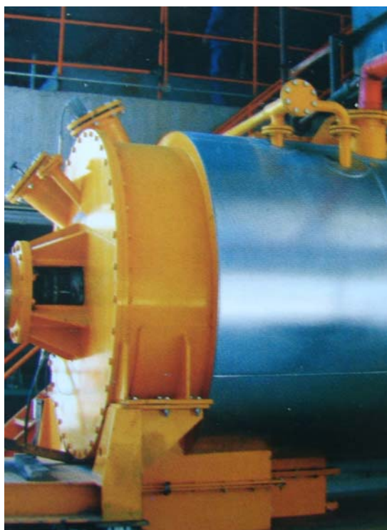
Figure 37: The real fly ash processing system.
