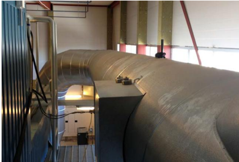
Figure 3: Skien bio boiler
