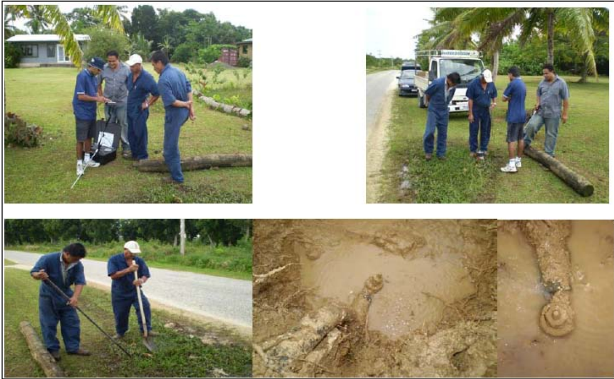
Figure 31: Leak detection exercise in Niue (Source: Author, 2007)
