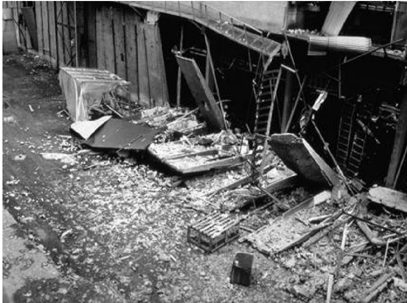
Figure 1.1: A photograph from the hydrogen gas explosion that occurred at a Norwegian ammonia plant (Norsk Hydro Ammonia NI) in 1985 [22].
