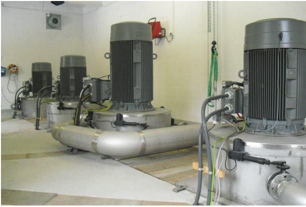
Figure 7: The four generator units in Sagbekken 2 and 3
