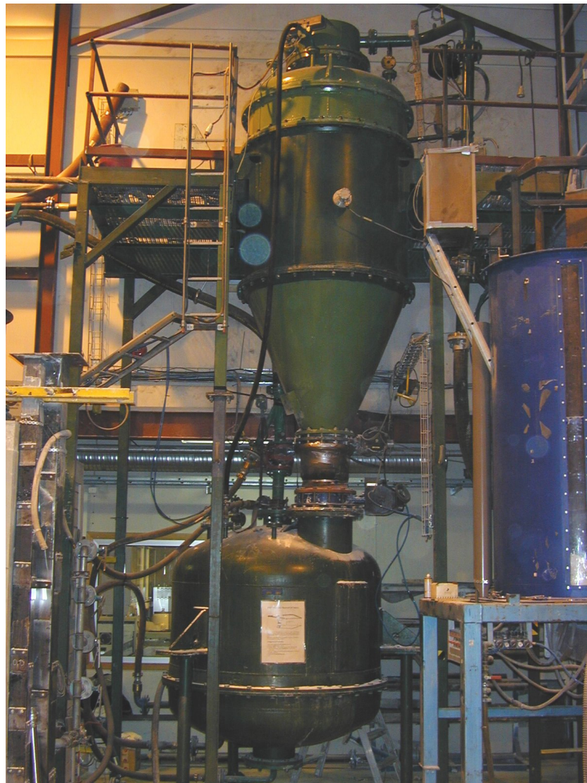
Figure 3-4: The blow tank and the receiving tank.
