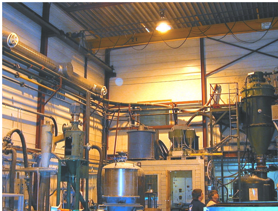
Figure 3-5: A part of the conveying pipeline.
