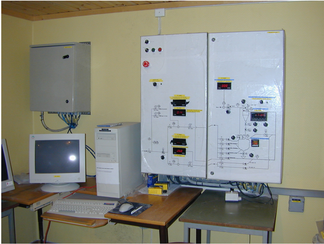
Figure 3-2: The arrangement of control panel and PC inside the control room.
