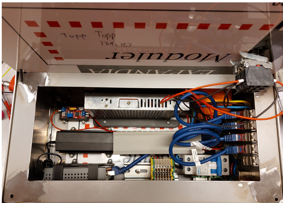
Figure 9.26: Inside the Power Supply box seen from above.
