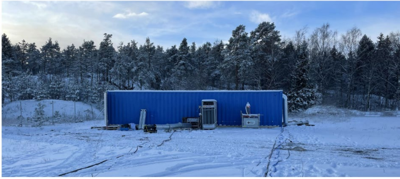
Figure 3.19: 40 ft ISO container with installed equipment and instrumentation.
