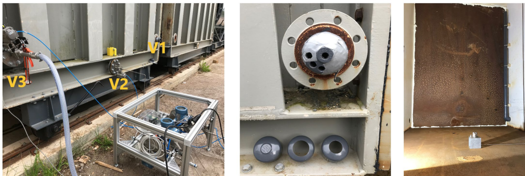
Figure 3.5: Pictures of vents on the front wall (left), ventilation assembly (middle), and the nozzle and PVC pipe-vent outlet inside the explosive chamber (right).
