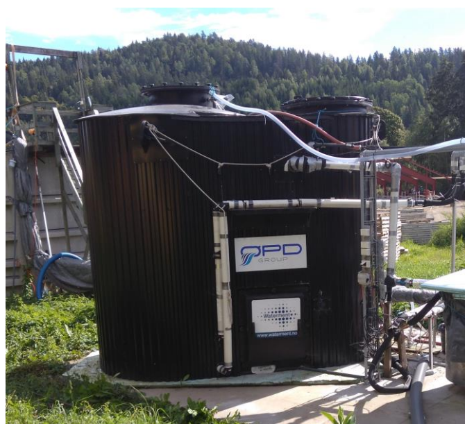
Figure 3.1: Pilot ABR reactor where samples were regularly investigated and reactor conditions monitored.
