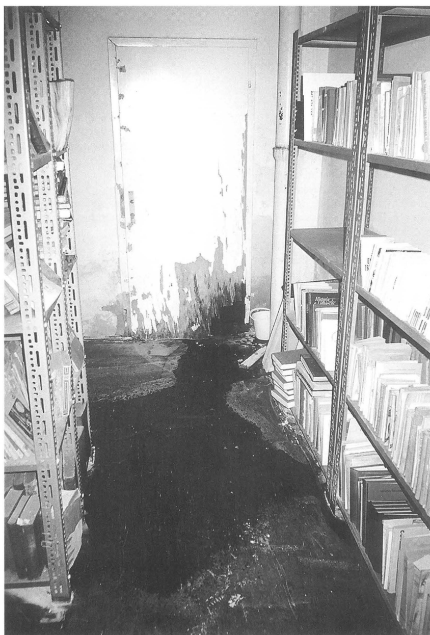
Serious water damages in the main library of Skanderaj located within the House of Culture.
